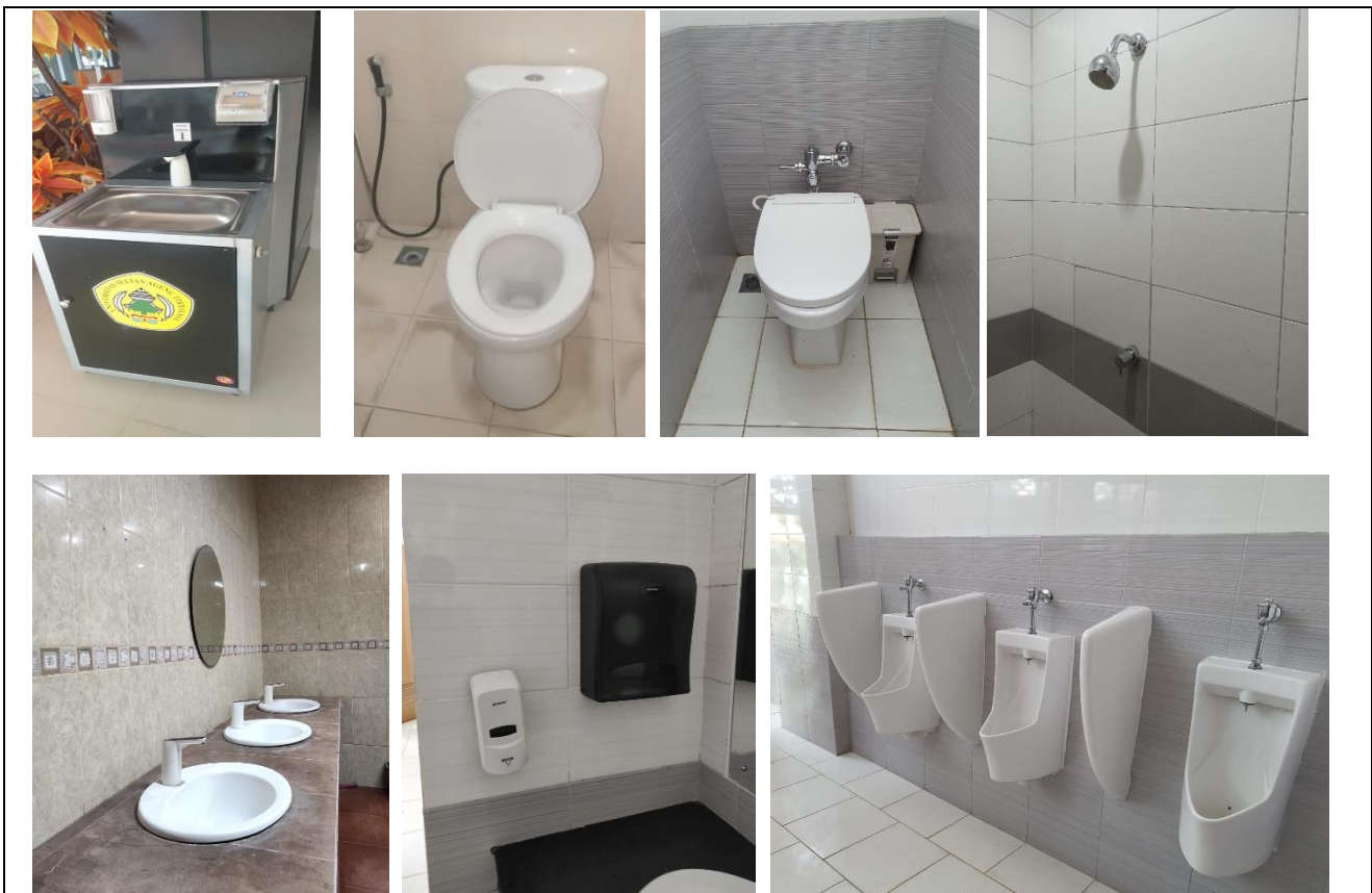
Figure 4.10 The Use of water-saving equipment
