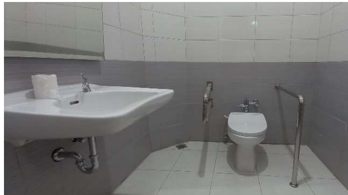
Wheelchair Track Facilities For Disabled And Disabled Toilets
