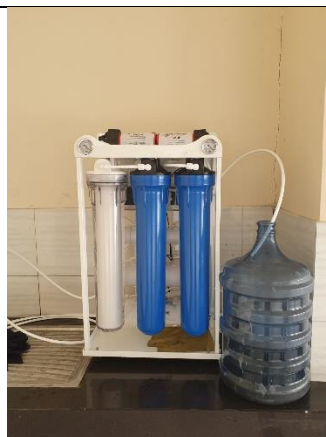
Figure 4.12 Tap Water facilities for ready to drink water
