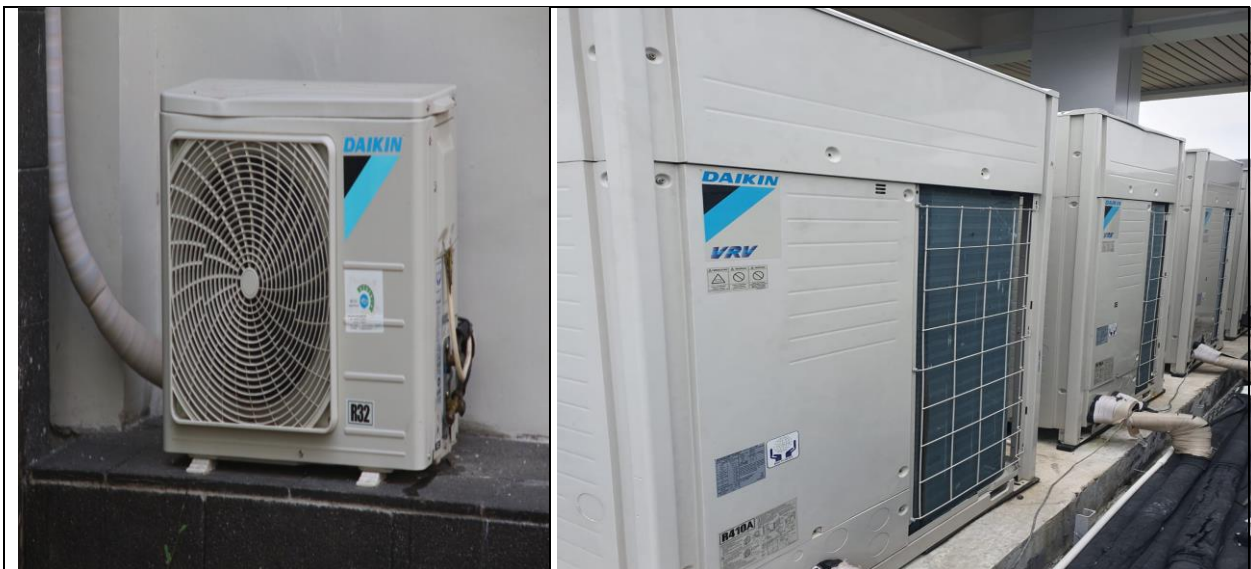
Example of Air Conditioning Inverter and VRV system (Campus E Universitas Sultan Ageng Tirtayasa)
