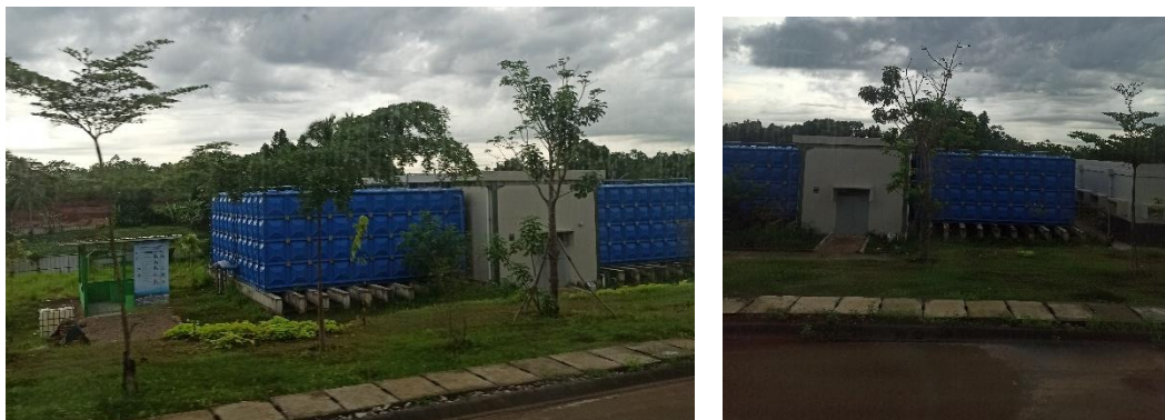
Figure 4.8 Water Treatment in Power House Area Untirta Sindang Sari
