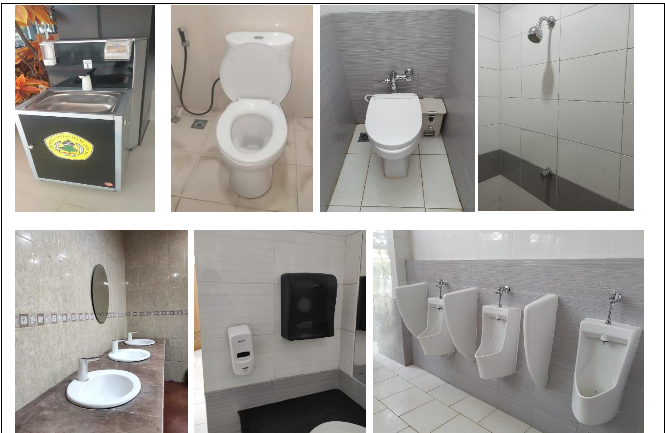
Figure 4.10 The Use of water-saving equipment
