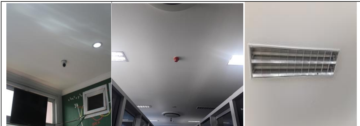
Example of LED light usage, Air Conditioning Inverter system (Campus B Universitas Sultan Ageng Tirtayasa)
