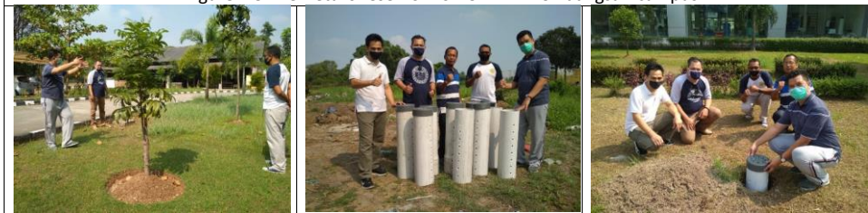
Figure 4.4 The Installation of bio pores and infiltration wells in the Engineering Faculty campus
