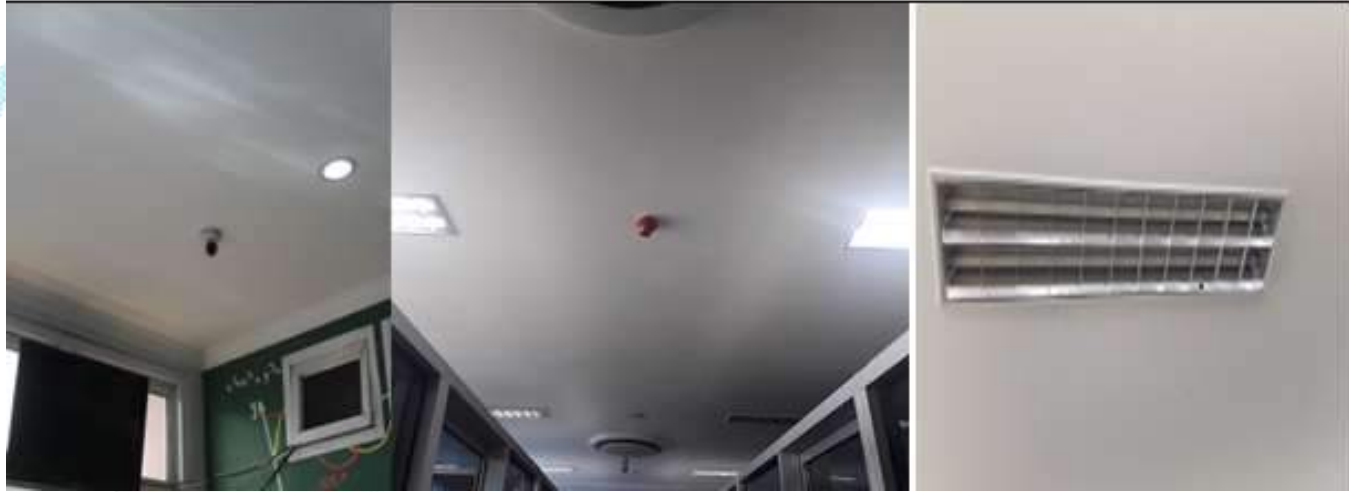
Example of LED light usage, Air Conditioning Inverter system for green building and energy saving
